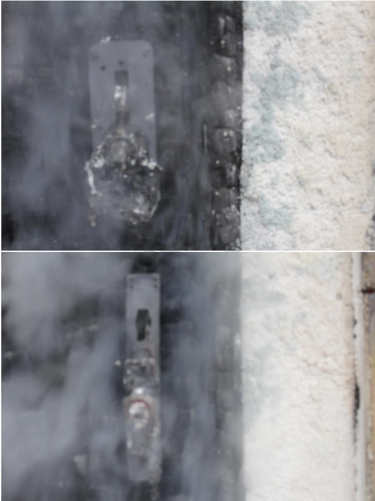
Figure 27 – Latch mechanism after the test (Still engaged)
